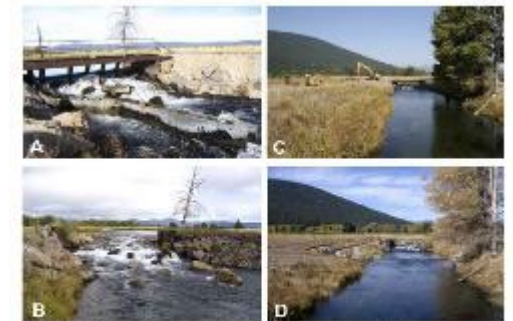
Figure 9-16: Photos of the river site showing the main channel diversion before construction (A) and to allow its replacement with a rock wall during the project (B), as well as showing the entire main channel before construction (C) and following replacement of diversion structure, channel roughening, and the addition of a fish bypass on the left following construction (D). Photos reproduced with permission from Trout Unlimited.
